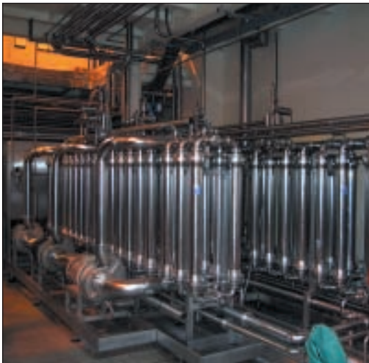
Cross-flow filters at Mathew Clark.
